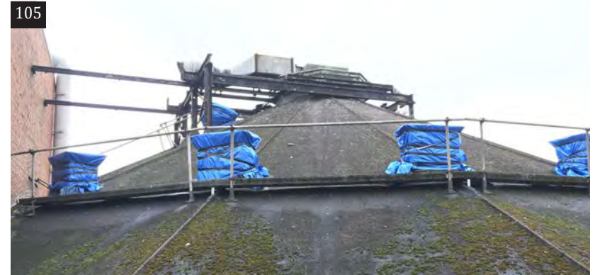
105: The sliding ventilator track on top of the dome is believed to be one of only four left in the country, the others being at the Apollo Victoria in London, the Bristol Hippodrome and the Pavilion Theatre, Glasgow
